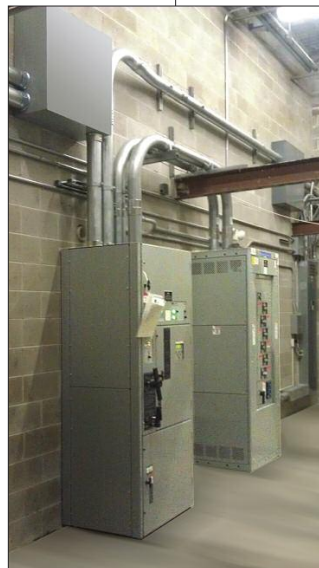
UNH Data Center ATS and Distribution Switchboard
