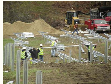
Patriot Solar Group, LLC was recently fined $1,000 by the Mass. DPL for unlicensed workers providing PV installations at this 3.5MW Solar farm in Southbridge, MA.
